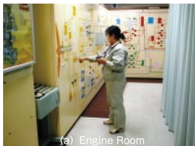
(a) Engine Room
